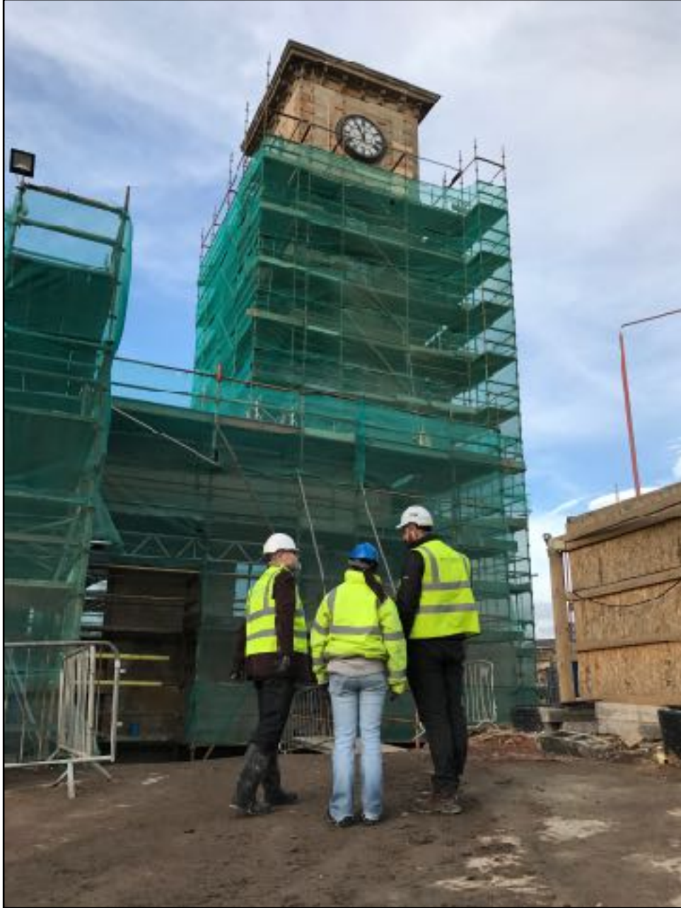
© GCHT Site inspection visit at the Pump House, Comprehensive building repair to reuse empty building, GCHT £84,591 for project costs to £211,357
