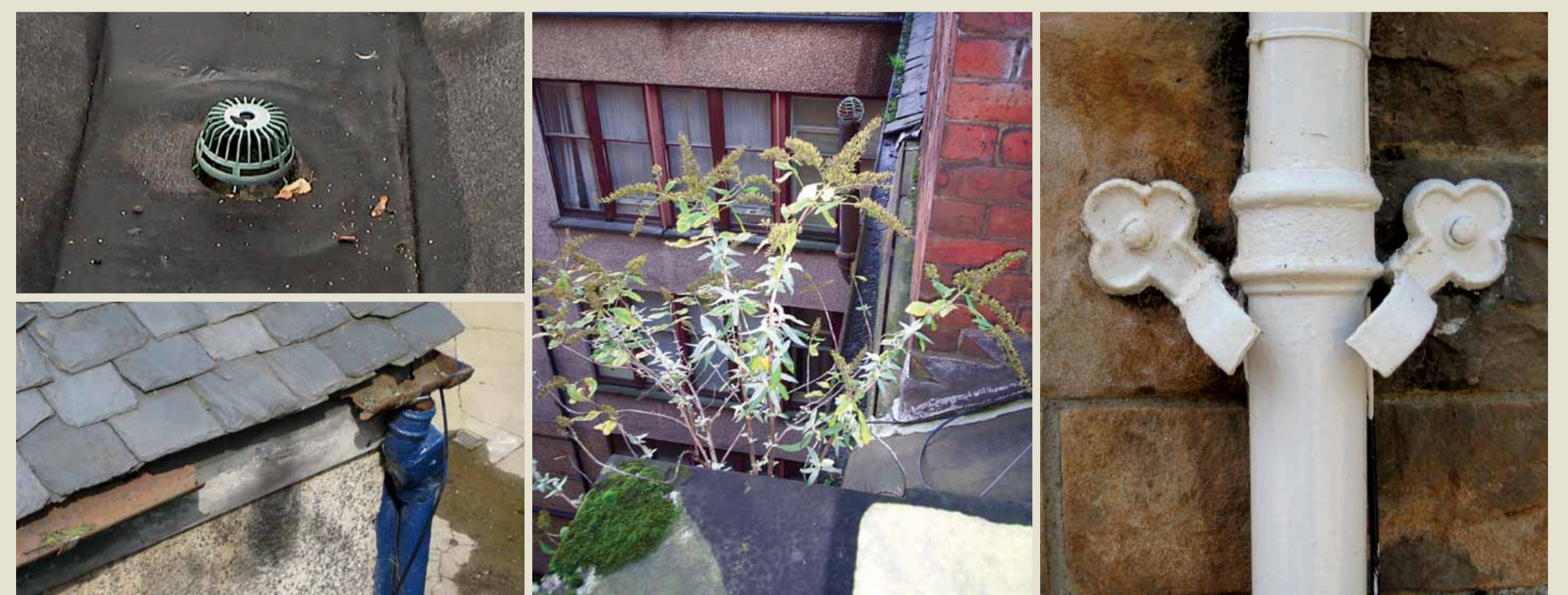
Balloon coverings will keep leaves and debris from blocking downpipes. Gutters should be cleared regularly to prevent plant growth and any damaged sections replaced. Victorian cast iron manufacturers in Glasgow were famous for their decorative embellishments.
